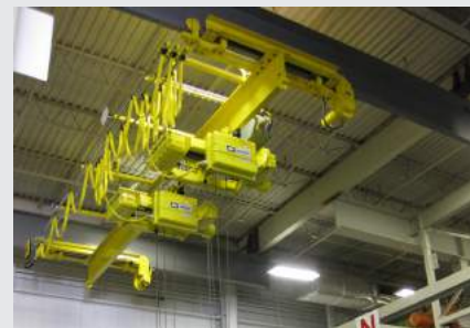
Louden crane with Speedway hoists.
